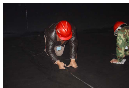
Figure 6. Install clipping in the demineralized water storage tank 图 6. 水箱内部进行安装剪裁
