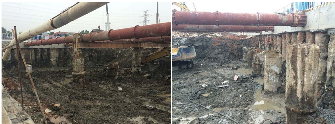
Figure 2. Support pile and steel support in U4 图 2. U4 段的支护桩及钢支撑
