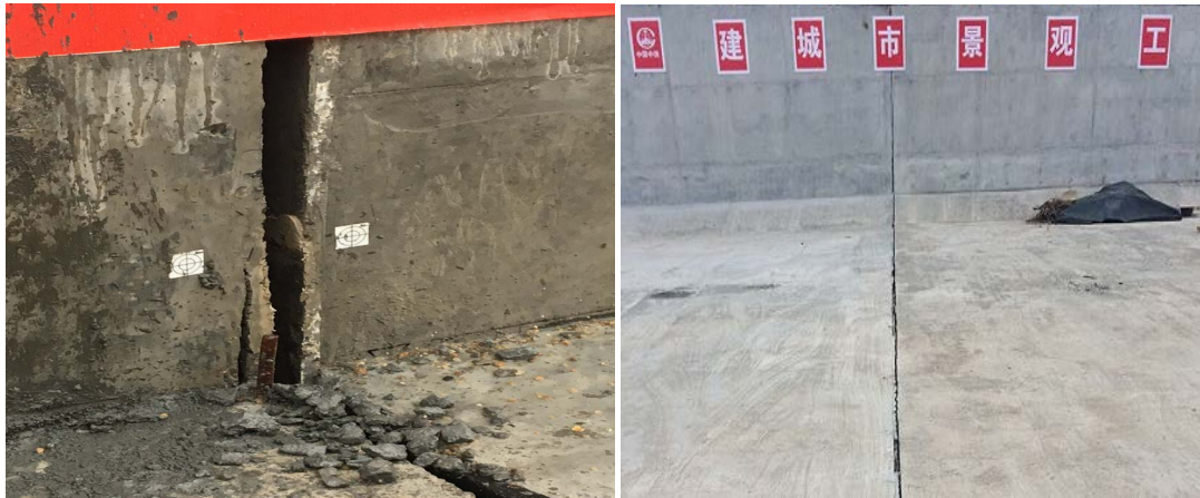
Figure 1. Crack between side wall and floor in U2 and U3 图 1. U2 和 U3 段侧壁和底板间裂缝
