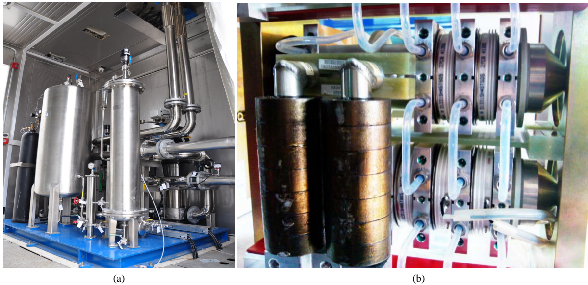
Figure 3. The main engine of the water cooling system 图 3. 水冷系统主机
