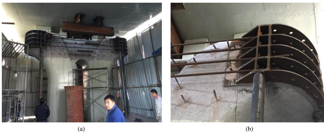
Figure 6. Reinforcement site: (a) Integral; (b) Steel anchor box 图 6. 加固现场。(a) 整体；(b) 钢锚箱
