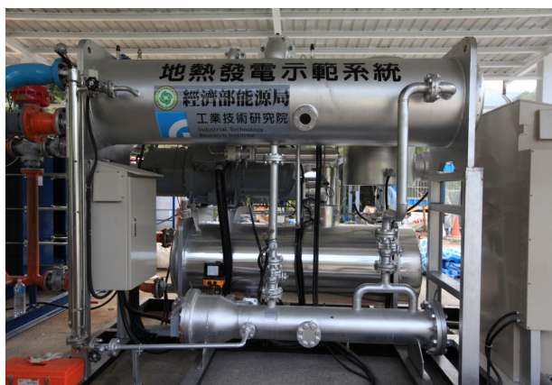
Figure 4. The 60 kW ORC generating system developed by ITRI installed at Chinsuei Yilan for geothermal power application 图 4. 工业技术研究院安装在宜兰县清水地热区的 60 kW 有机朗肯循环发电系统
